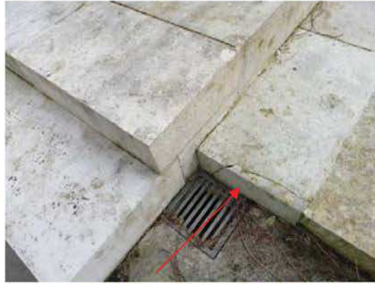
Picture 12. Damage to stone
