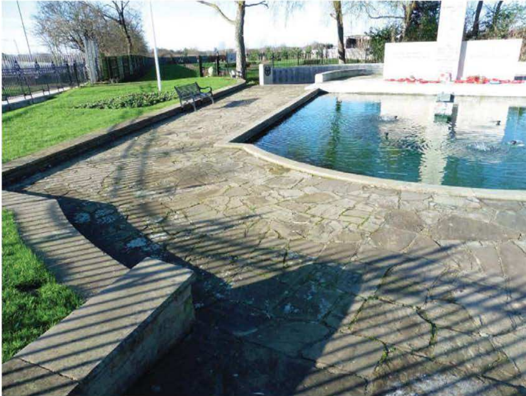
Picture 7. Open joints to York paving and copings
