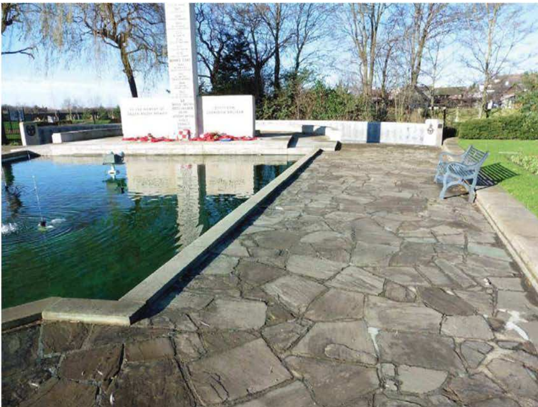
Picture 6. Open joints to York paving with previous patching
