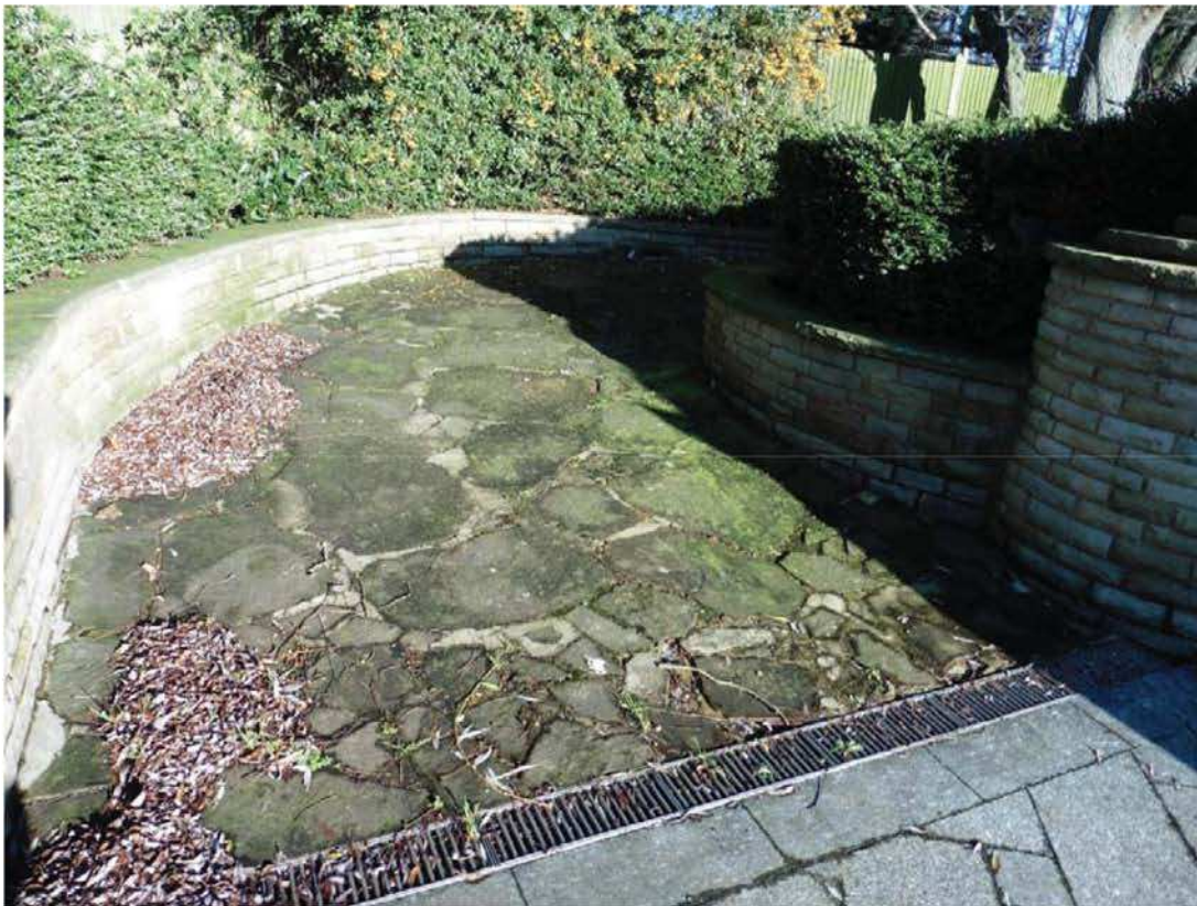
Picture 4. Showing previous patching and further deterioration to York paving
