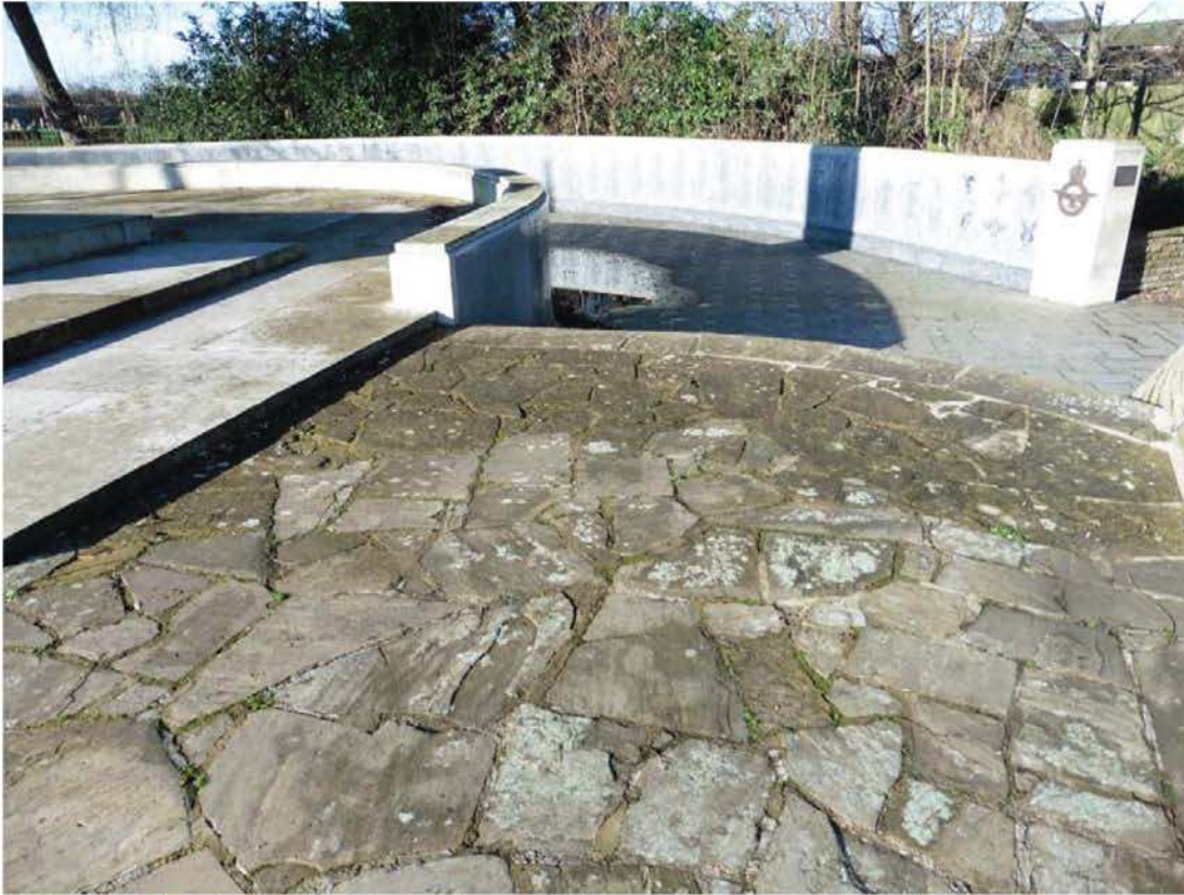
Picture 5. Showing York paving with open joints and with some vegetative growth
