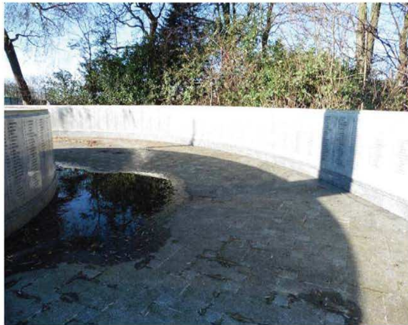
Picture 2. Granite section showing ponding
