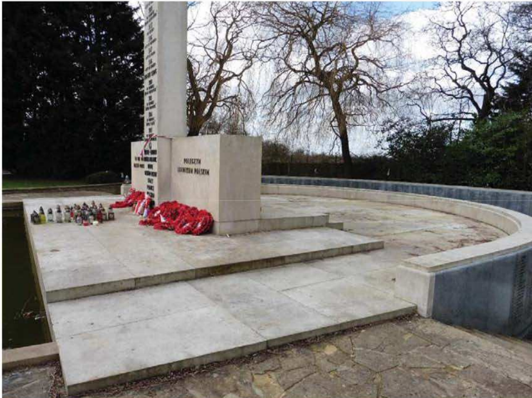
Picture 10. Showing position of damage in close up in picture 11
